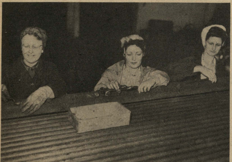
Boilermakers Swan Island has thousands of women boilermakers, but these are the only three who actually help make boilers. Shown here tightening bolts on air heater are, left to right, L. S. Kilmer, Ann Grifinn and M. R. Worster of Boiler Erection department. (Swan Island photo)
