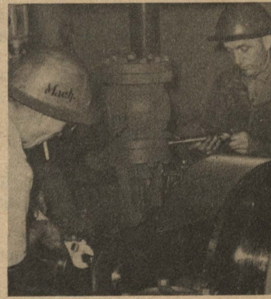
7. Gear cover has been lifted, exposing reduction gear. Tooth contact of gear must be set to within .0005 of an inch. At left is Leadman Bronson.
