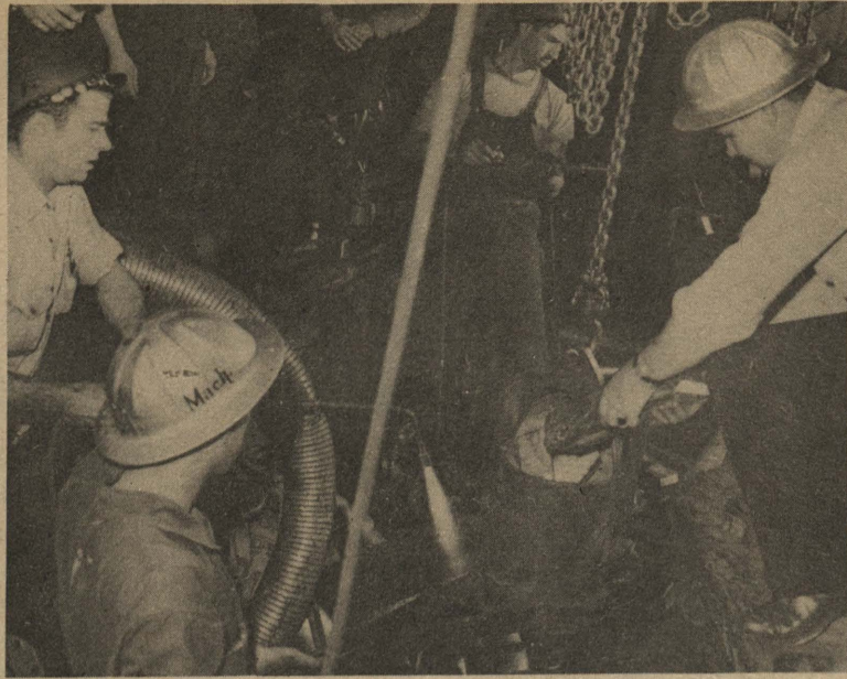
2. Type metal bars are melted by heaters in preparation for pouring of chocks under thrust bearing. At left, J. Millner, with torch. Cates holds melting pot while Foreman Smith adds another bar. At center back, Leadman Hunt heats a second pot of metal.
