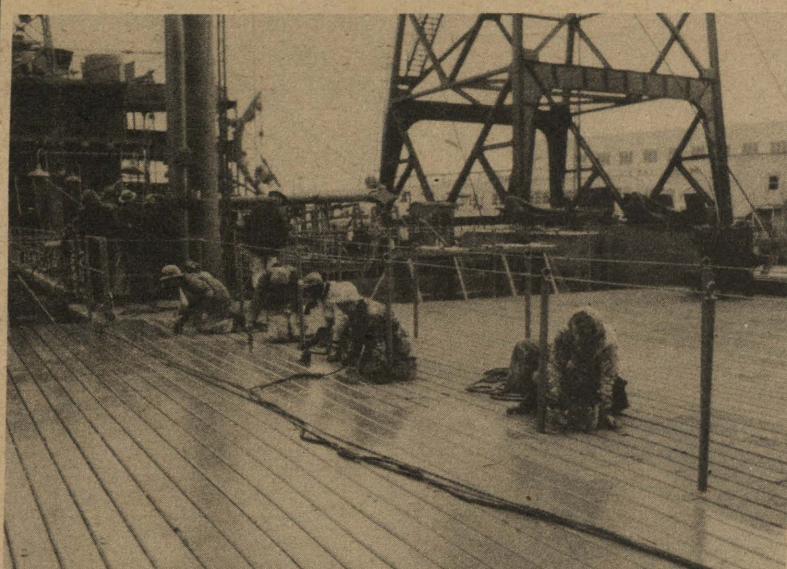
Last Coat Day shift painters slap last coat of deck paint on Fleet Oiler 106 day before its trial run. Electricians are busy at mast. (Swan Island Photo)
