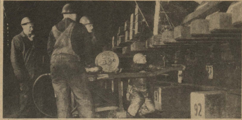
8:30 a.m. Grease irons are removed allowing sliding ways to contact standing ways. Shown here are F. J. German, Dick Lahti, John Johnson and Joe La Gregor. The half-inch iron straps were previously placed between the standing ways and the sliding ways at regular intervals.
