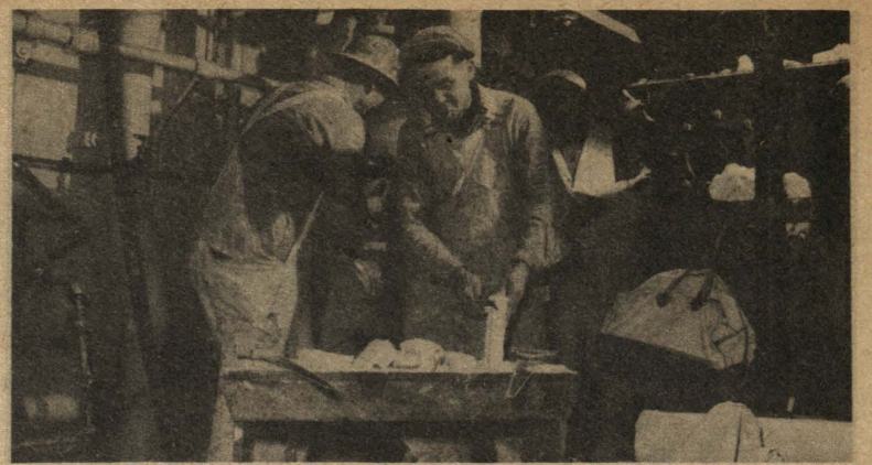
Asbestos Men Charles Snyder, Phil Smith and Hy Pifer fit asbestos insulation on boiler room pipes of a Swan Island tanker at the Outfitting dock. (Swan Island photo)
