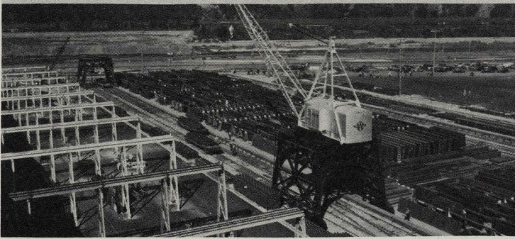
Cranes from the Plate Shop travel out on these extensions at the left, picking up plates from the storage area (center).
