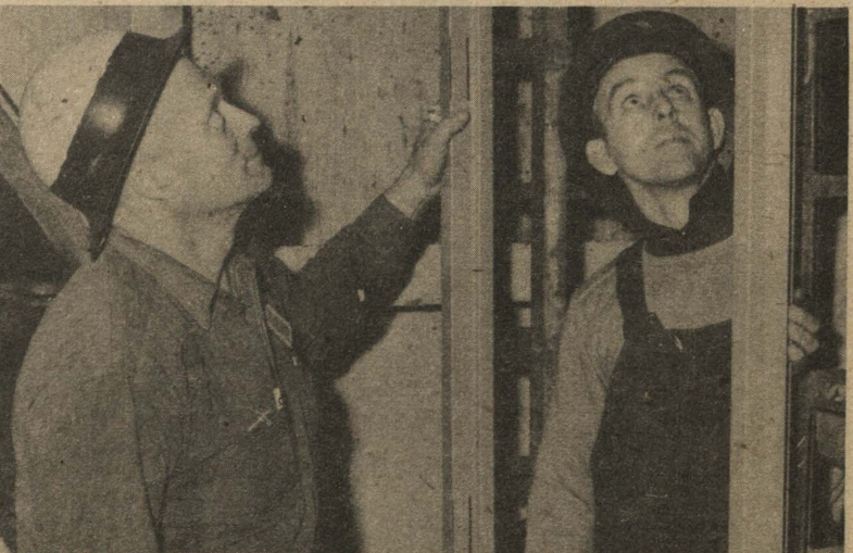
Work With Metal Two Vancouver Bucklerites hang one of the 185 metal door frames which go aboard an aircraft carrier. Buckler outfitters at Vancouver deal exclusively with metal, those at Oregon Ship handle wood joinery.
