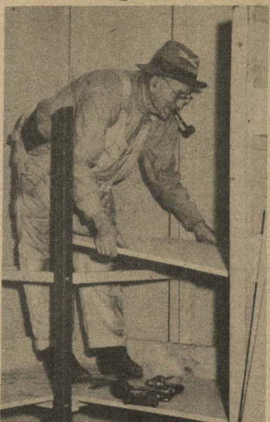
O. B. "Bill" Dillinham, O.S.C. Buckler-Chapman joiner, puts in a section of shelving in a dry stores space, for canned goods storage.
