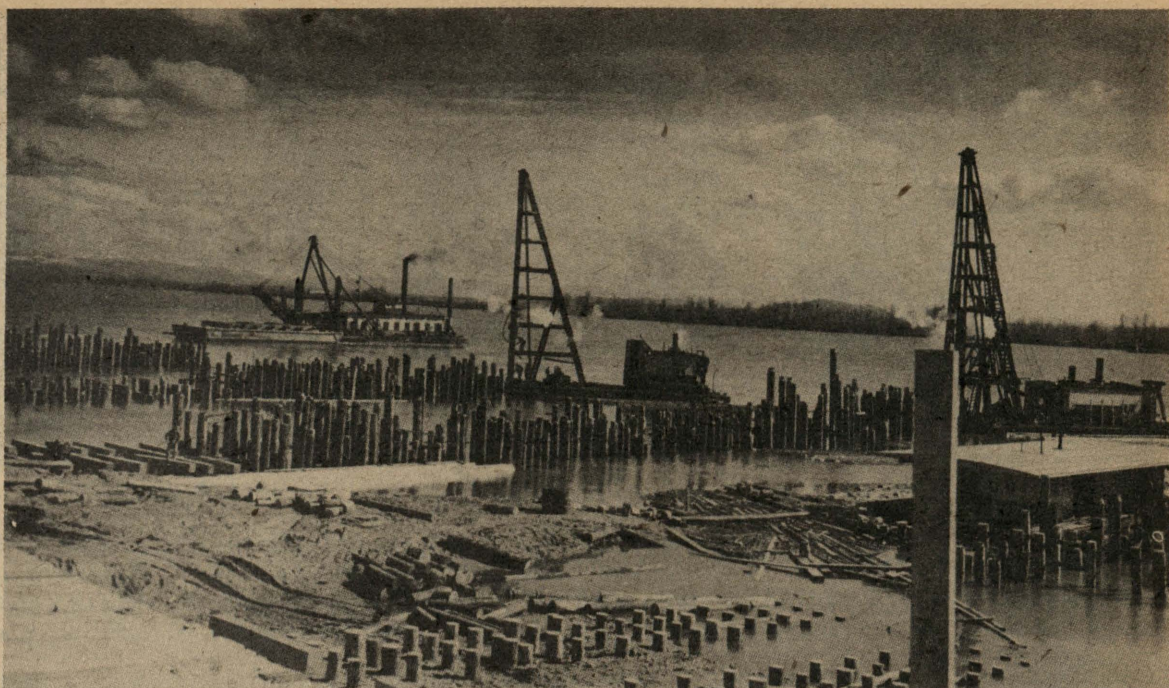
Three year club members went to work at Kaiser company's Vancouver yard when pile drivers were busy on the earliest construction on the ways, as seen in the picture above, taken March 15, 1942. There were only 1000 employes at that time.
