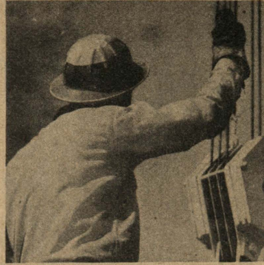
Hoist! Carl Going, Oregon leadman, signals the crane operator that the load, or the boom, is ready to go up. Certain riggers on each crew may give signals.
